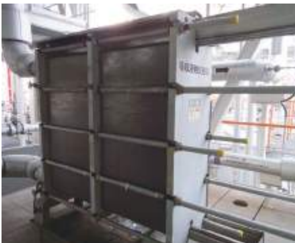
CO 2 recovery, desulfurization plant solution heat exchange
