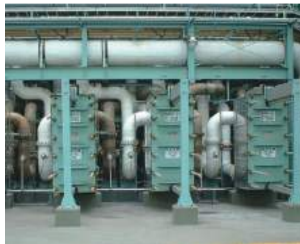
Sulfuric acid, electrolytic plating cooling
