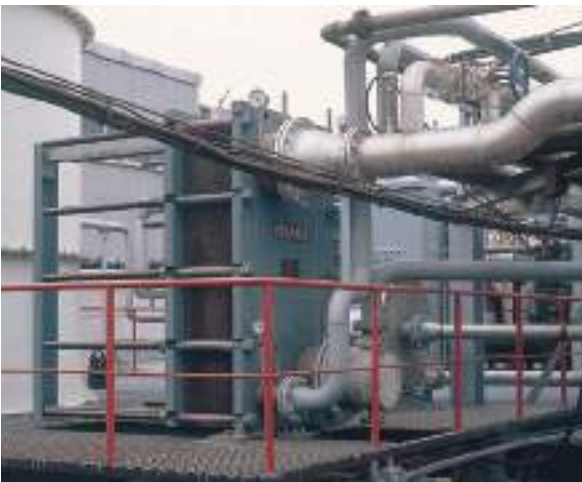
Solvent recovery, exhaust gas cooling
