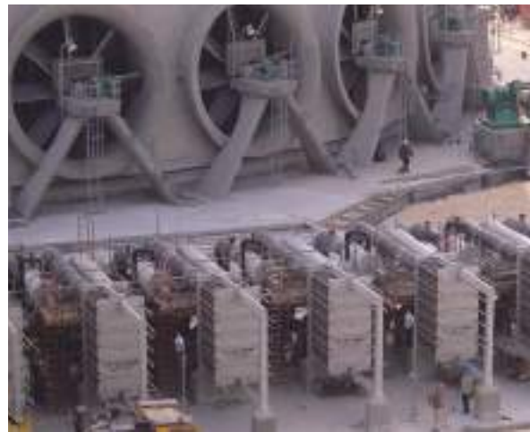
Central cooling system
