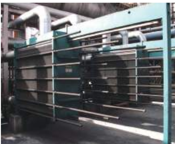
Blast furnace cooling, continuous casting equipment cooling, COG, various plating fluid cooling
